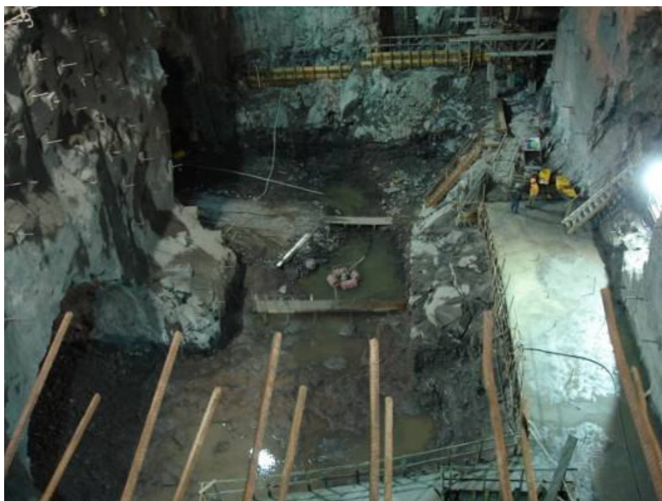
Figure 3.2 – Power House – Turbines well – Source: CERAN
